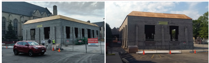
Above are images and an artist's rendering of Kyte Hall, a multipurpose space that was recently built at St. Vincent Ferrer parish that will also serve as a lunchroom for the parish's school.
