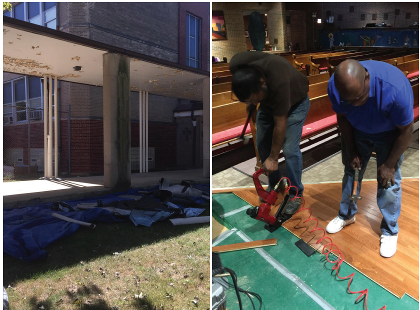
The To Teach Who Christ Is campaign has provided Holy Name of Mary Parish with funds to execute internal and external renovation plans, including repairing the parish's roof and floors.
