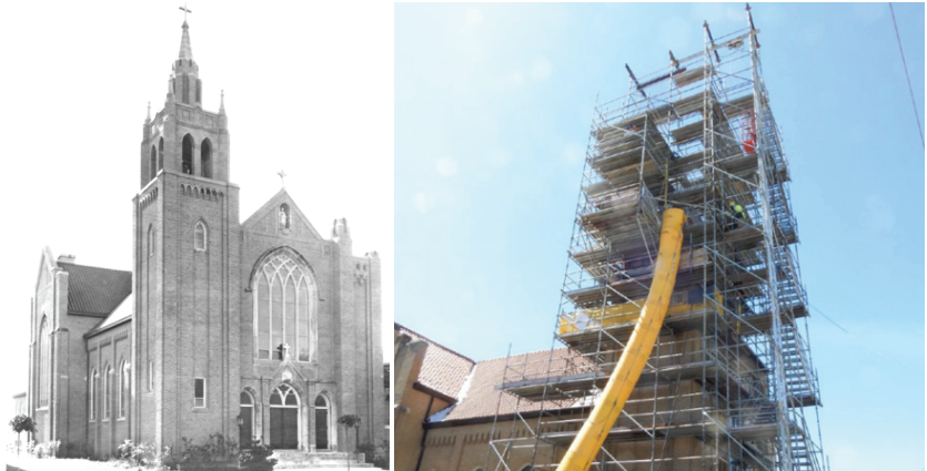
The new bell tower at St. Peter’s, which will be completed this summer, is being constructed with details from the original 1925 blueprints, and will bring the sound of a church bell to Volo and to neighboring areas.
